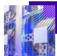
Aligned Data Centers' patented cooling technology, Delta 3 at the Phoenix 01/02/03 Data Center, United States
