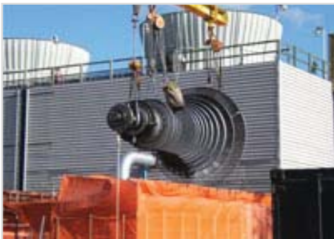
A crane lifts the turbine out of the Whitecourt plant for maintenance.
