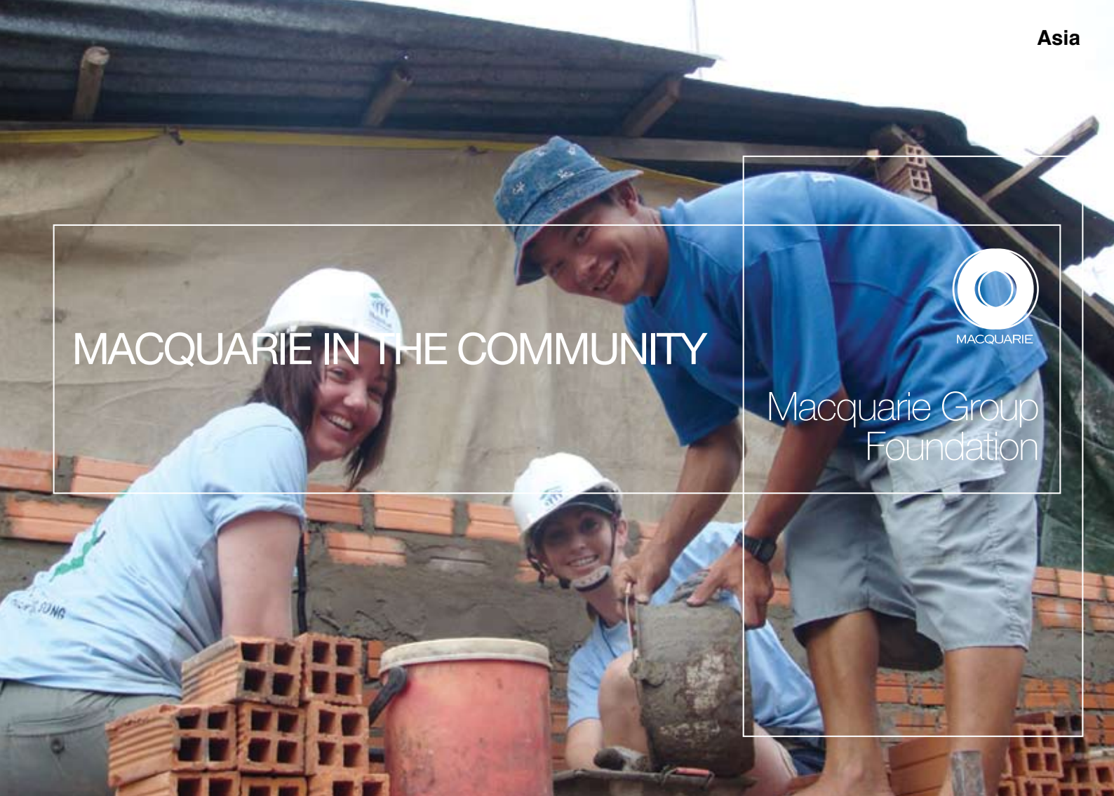
Tegan Higginbotham and Carinda Harris from MSG in Sydney building a home for a family in need in Vietnam.
